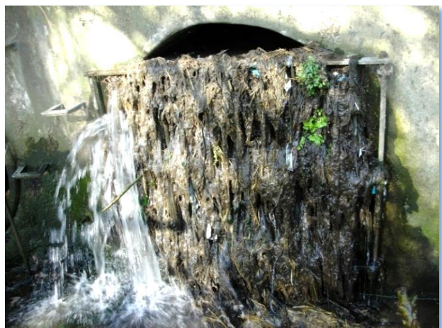
Asfordby Road rainwater outlet pictured in 2012 clogged with toilet waste, although it looks much the same today
